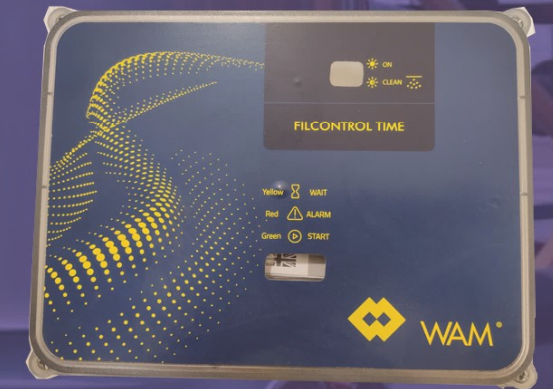
CONTROL PANEL - R03
